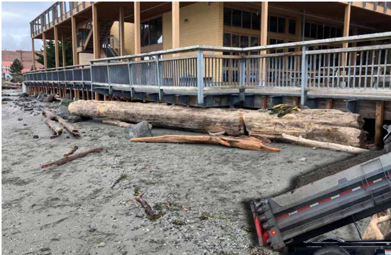
The log before it had been removed from under the Maritime Center's deck area. (Above right) The tug used to remove the log. (Right) A city vehicle dropping off cobble to fill around the log. Photos courtesy of Port of Port Townsend
